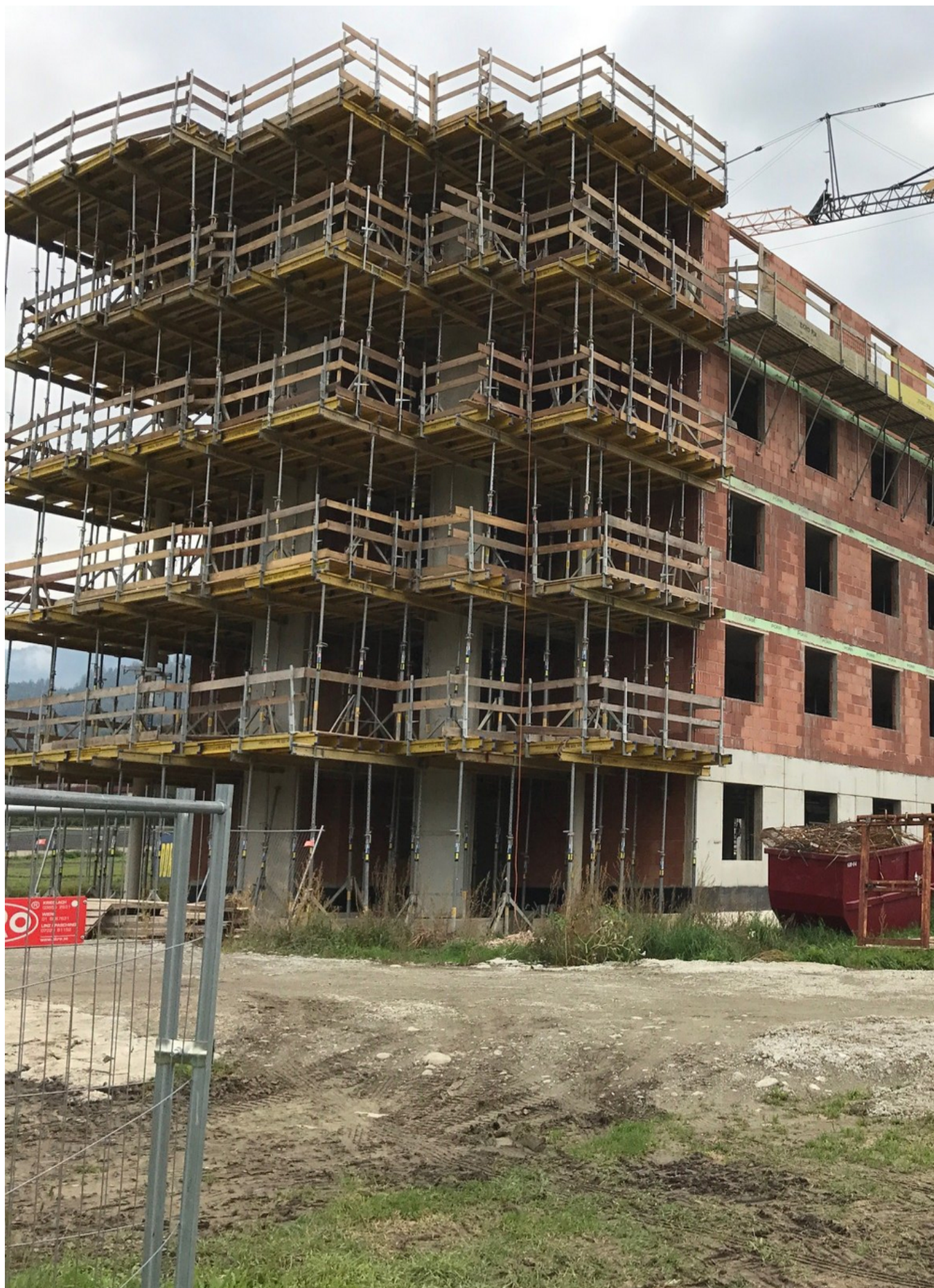
The external walls and the load-bearing walls in the vicinity of the staircases are composed of vertical coring bricks. Source: PORR
