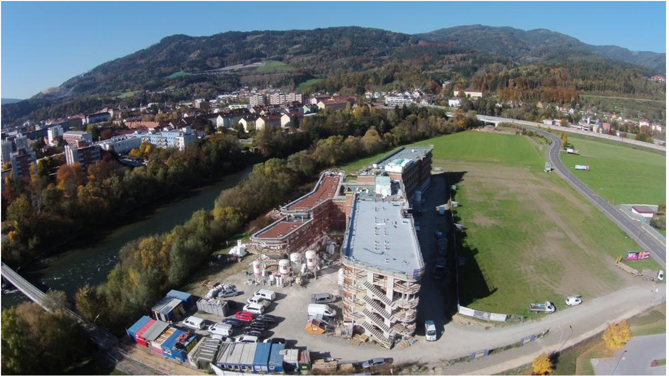
The building features flat roofs in all areas. The shorter of the two main building sections features an extensive green roof. Source: PORR
