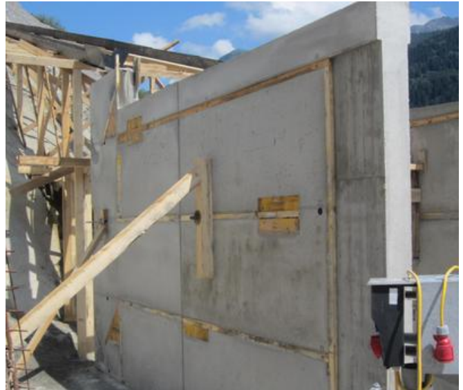
In the TB Stams concrete factory, a large-scale test was carried out to find a suitable concrete recipe for the concrete backfill. Source: GKI PRB consortium
