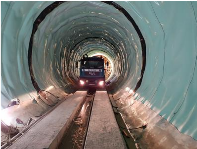
The sealing work was carried out in parallel with the concrete production, during night shifts. Source: GKI PRB consortium
