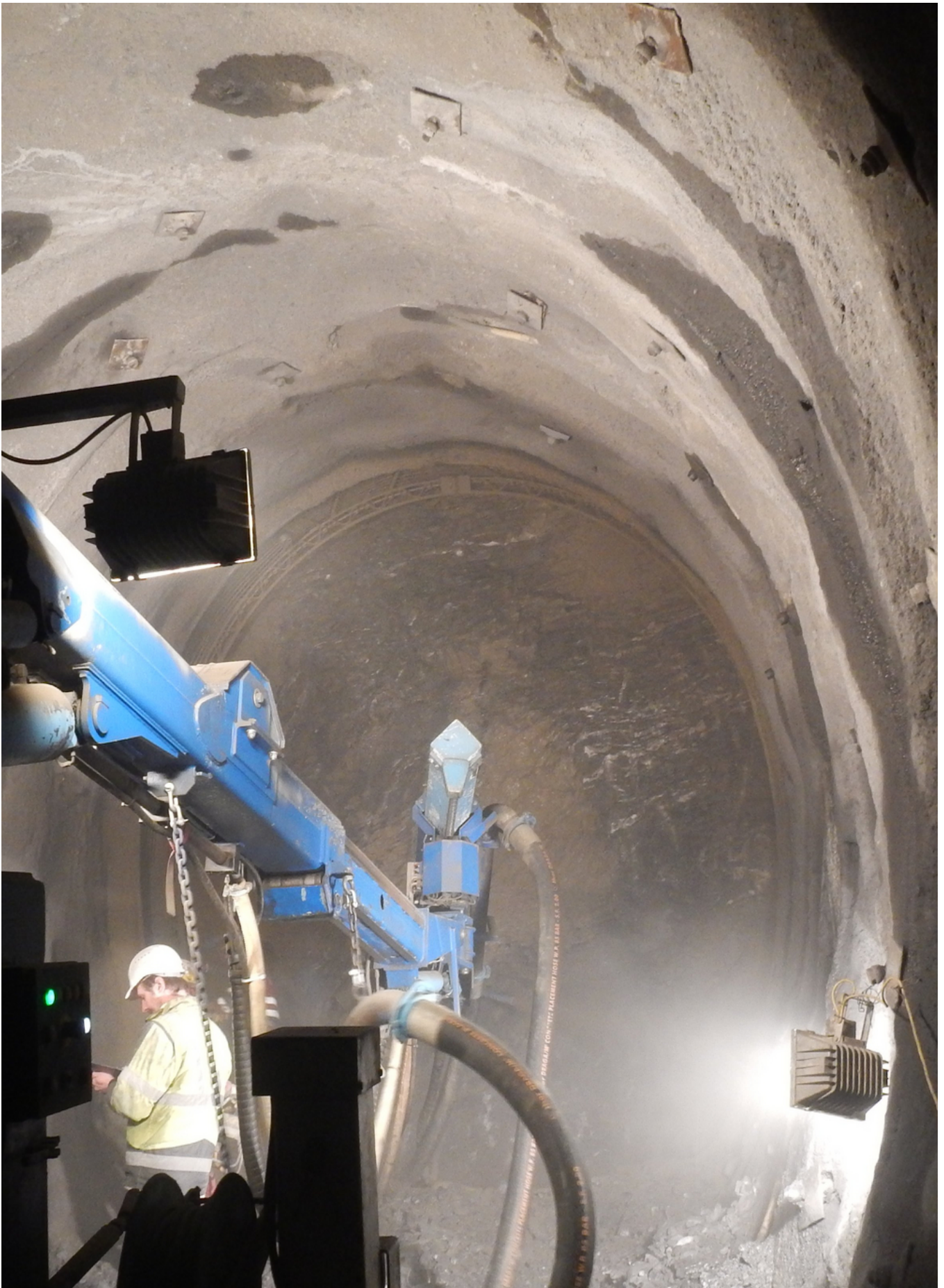
The tunnel boring work in the inclined shaft was given priority, so that the schedule could be met. Source: GKI PRB consortium
