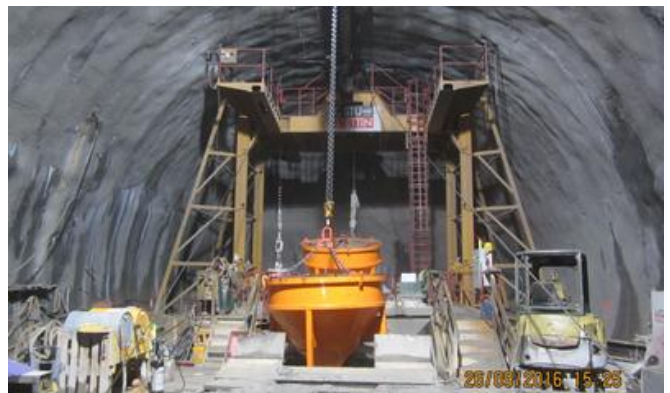
The working platform for the poured concrete was subsequently used as a platform for all the shaft work. Source: GKI PRB consortium
