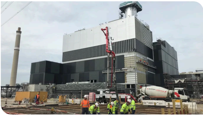
Concreting the outdoor storage area floor slab for the Marzahn combined heat and power station. Source: PORR/Fabian Hemauer
