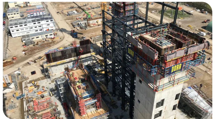
In an effort to meet weekly deadlines, the stairwells had to be heated and coated in frost protection mats over the weekends. Source: PORR/Fabian Hemaier
