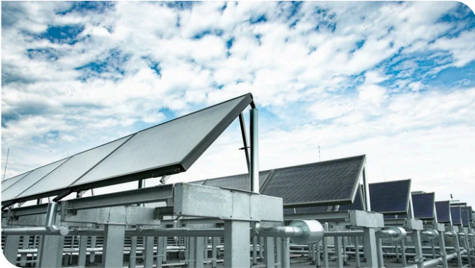
In order to increase the building's energy efficiency, a solar system was installed on the roof to heat water. Source: PORR
