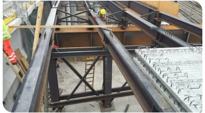
To create space for the construction site facilities and maintain ongoing traffic, the lanes were temporarily widened with the aid of composite steel bridges. Source: PORR
