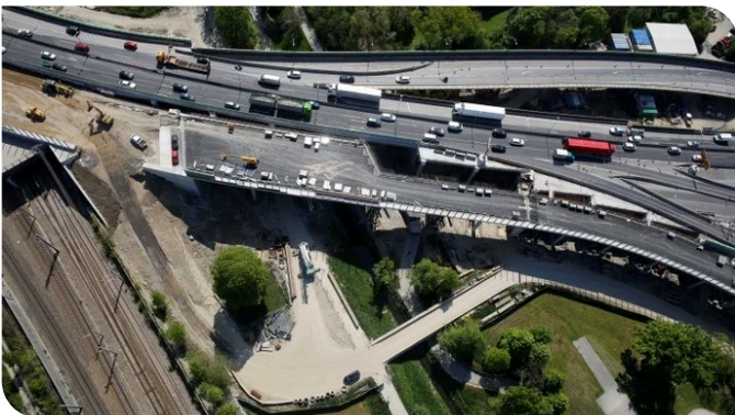
Several bridges were completely or partially rebuilt and an existing tunnel was backfilled. Source: PORR
