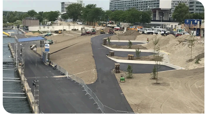
PORR erected several retaining walls featuring irregular curves along the embankment area. The largest retaining wall begins at the quay and ends at the top of the embankment (visible in the background). Source: PORR
