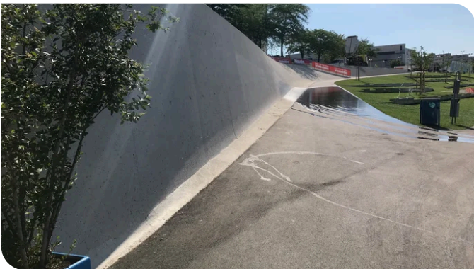
Custom-made formwork was needed to produce the exposed concrete surfaces. Source: PORR
